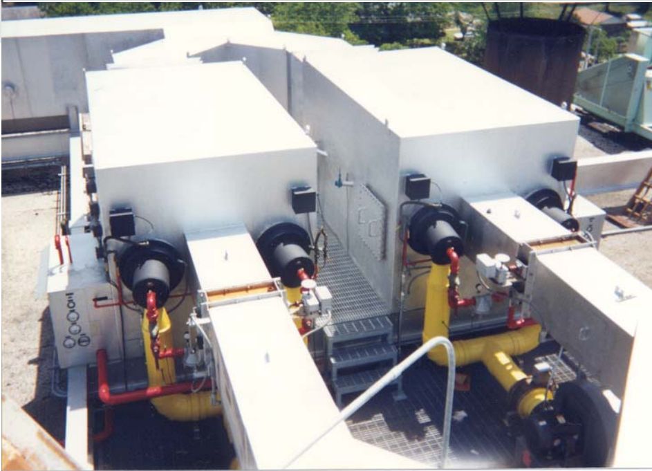
Waste fume incinerators for Escambia County Sewage Treatment Plant, Pensacola, Florida
